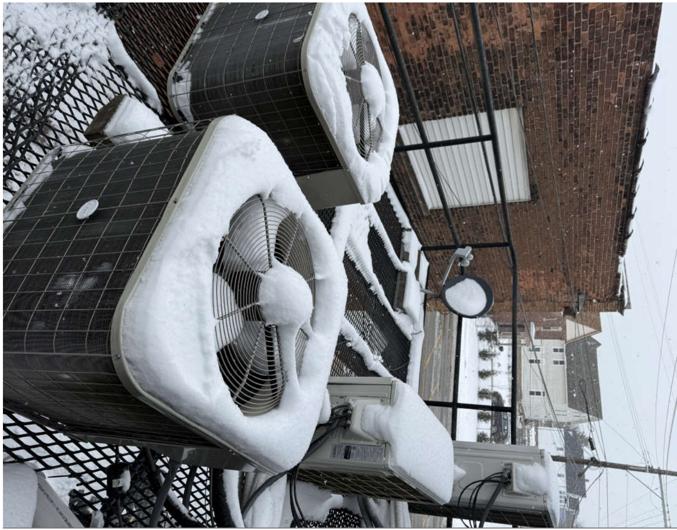
HVAC EQUIPMENT ON PLATFORM
