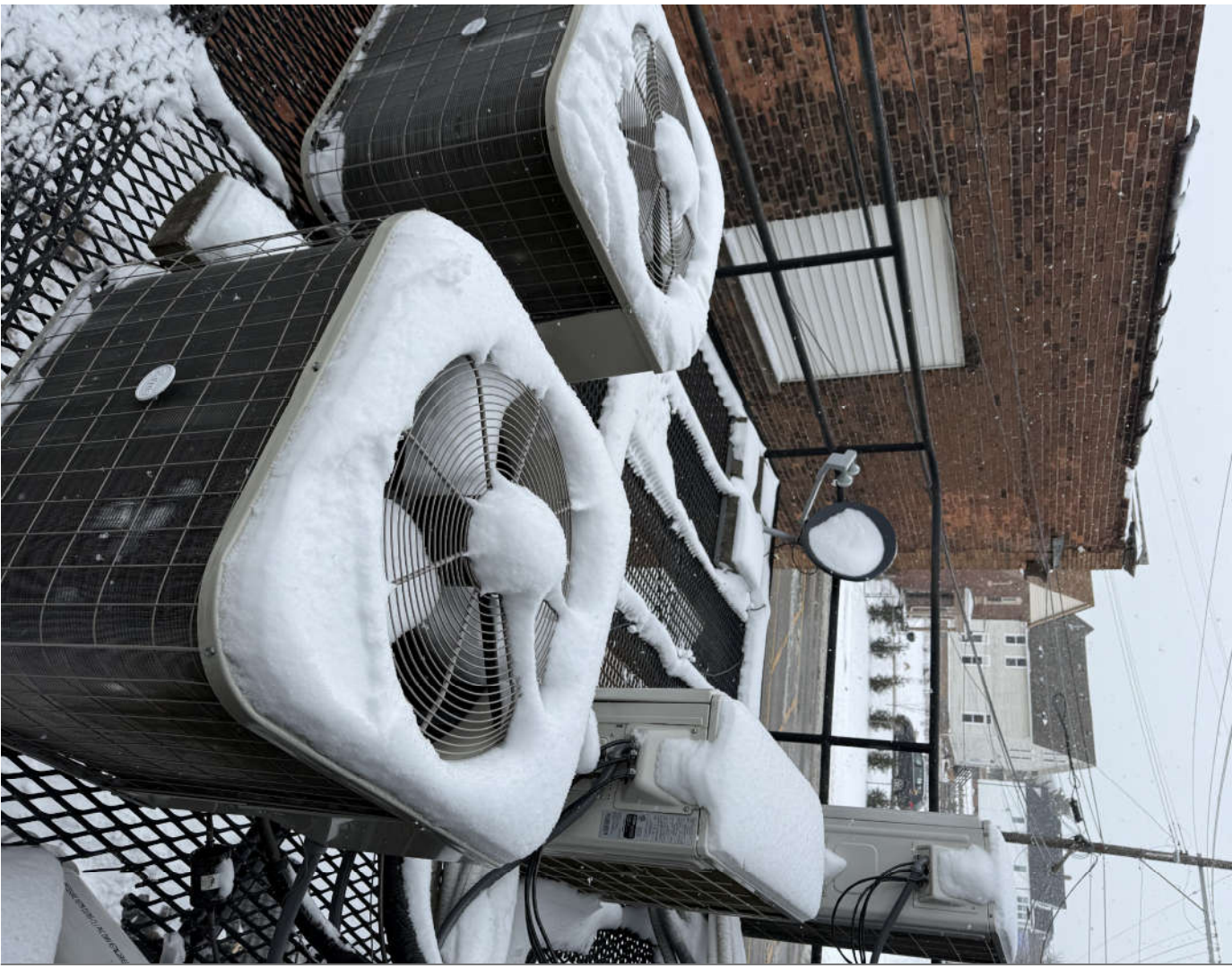
HVAC EQUIPMENT ON PLATFORM
