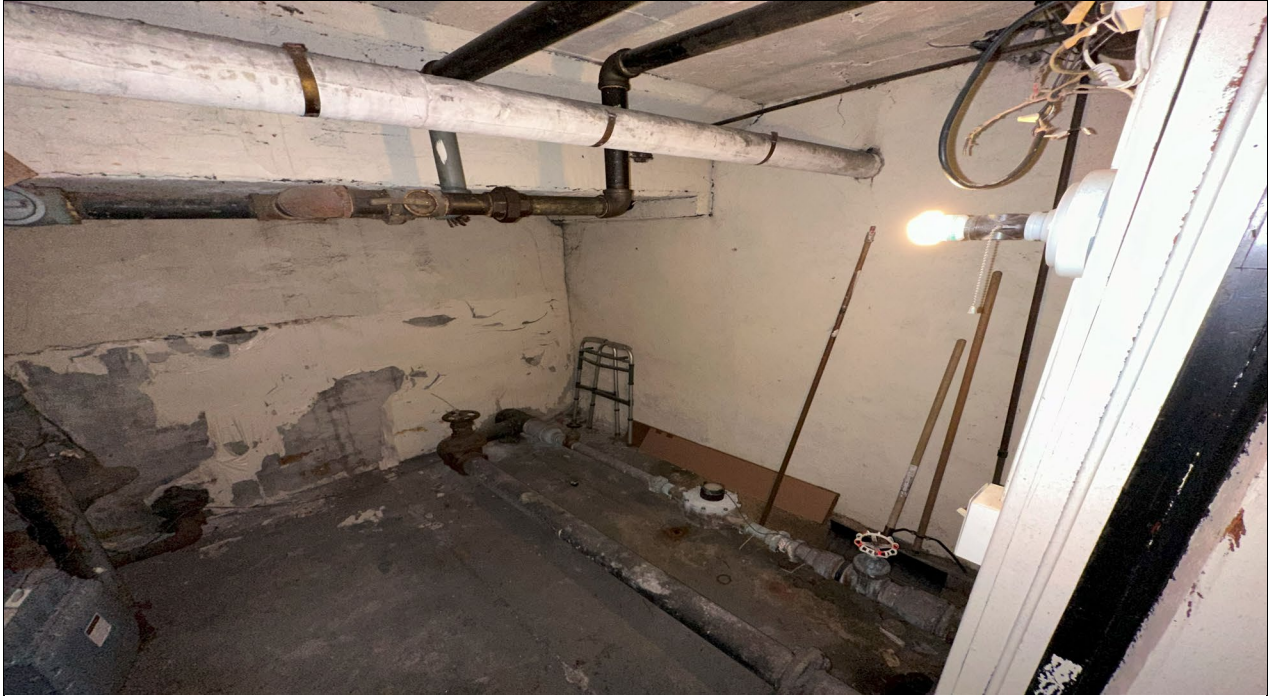
Photograph 17. 489 Henry Street Parcel: Meter room.
