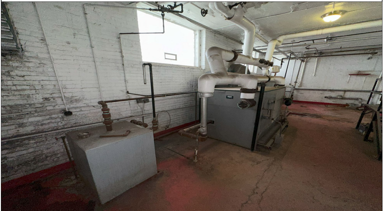
Photograph 20. 489 Henry Street Parcel: Boiler room.
