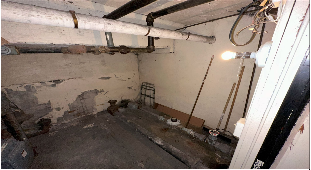
Photograph 17. 489 Henry Street Parcel: Meter room.
