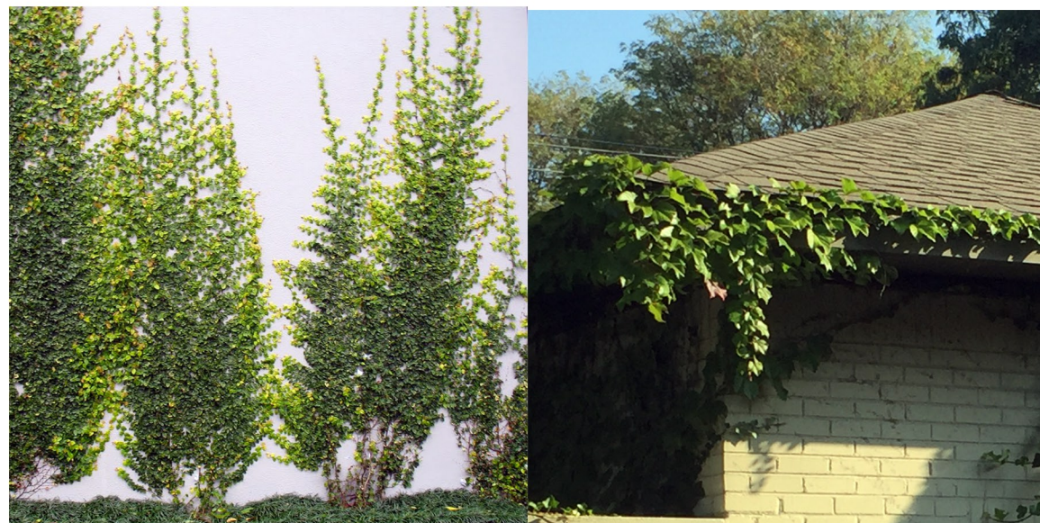
BOSTON IVY ON WALLS & GROWING UP ONTO BUILDING OVERHANG
