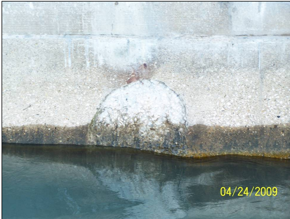
Photograph 93: View of Pier 4 Section Loss on South Face.
