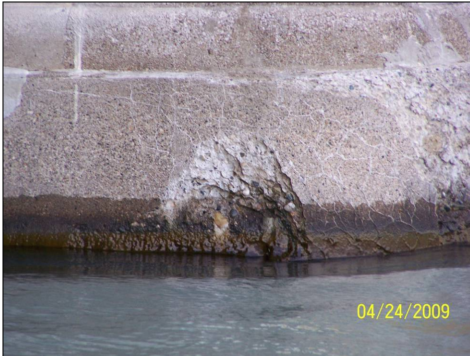
Photograph 107: View of Pier 18 Section Loss on North Face.
