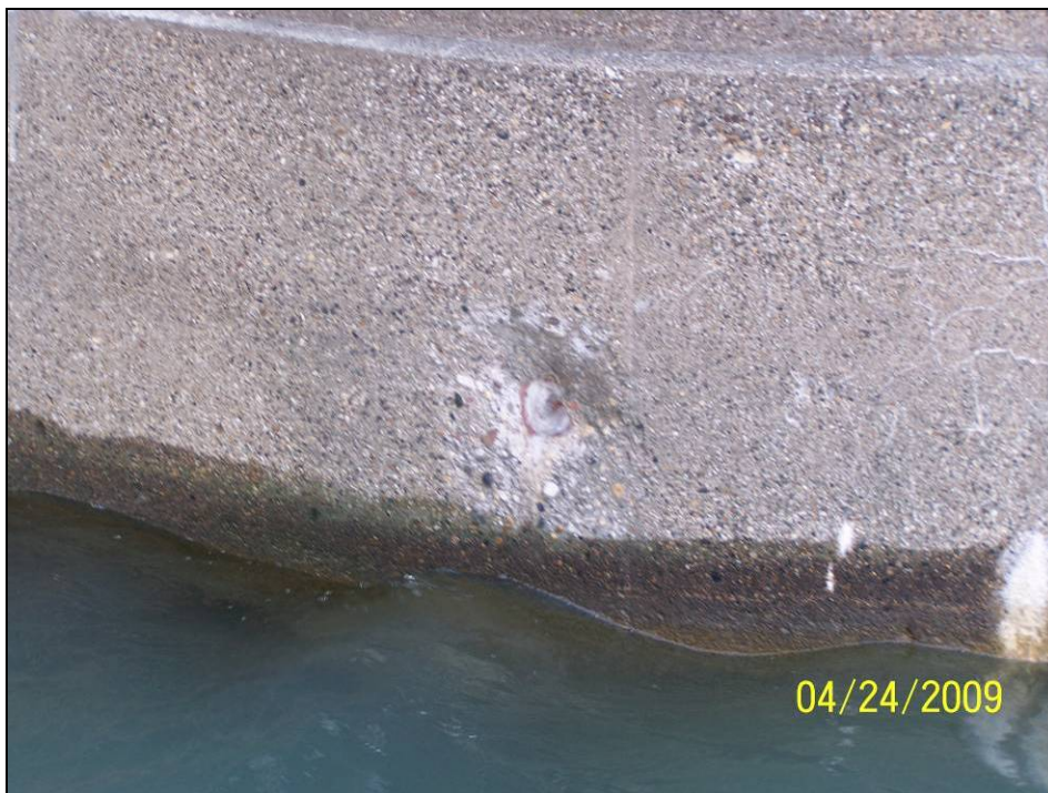
Photograph 90: View of Pier 1 Section Loss Near Northwest Corner.
