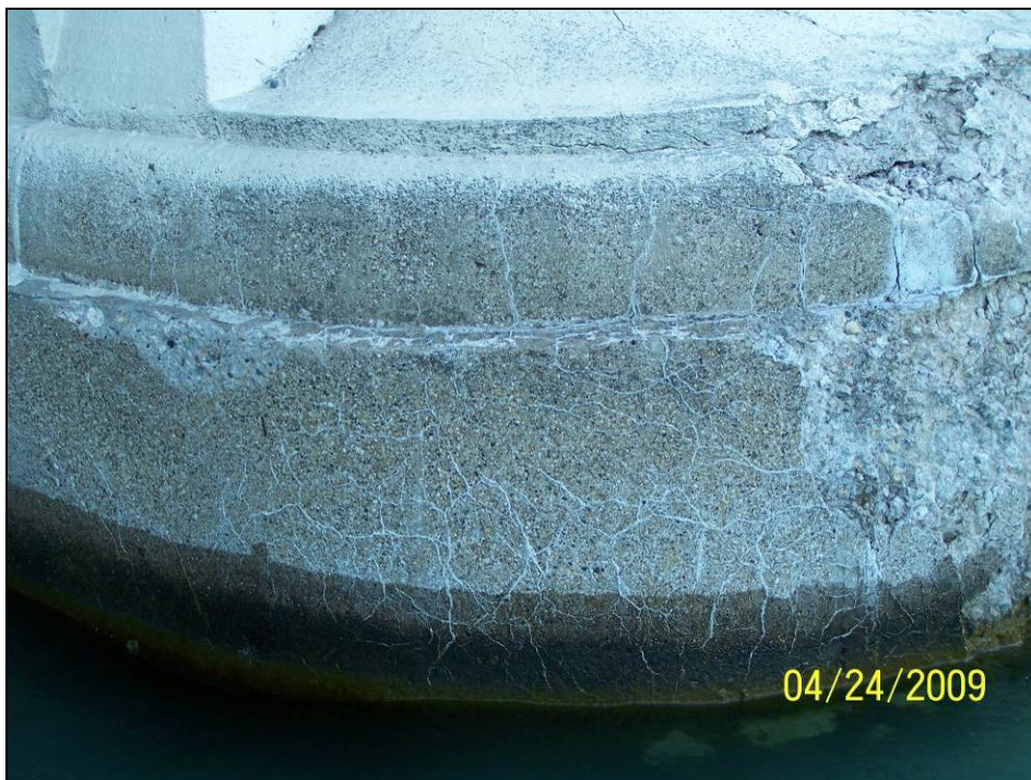
Photograph 106: View of Pier 17 Map Cracking on Downstream Nose.
