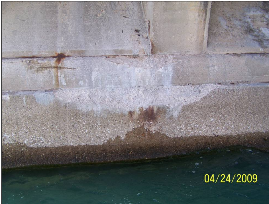
Photograph 97: View of Pier 10 Section Loss on North Face.
