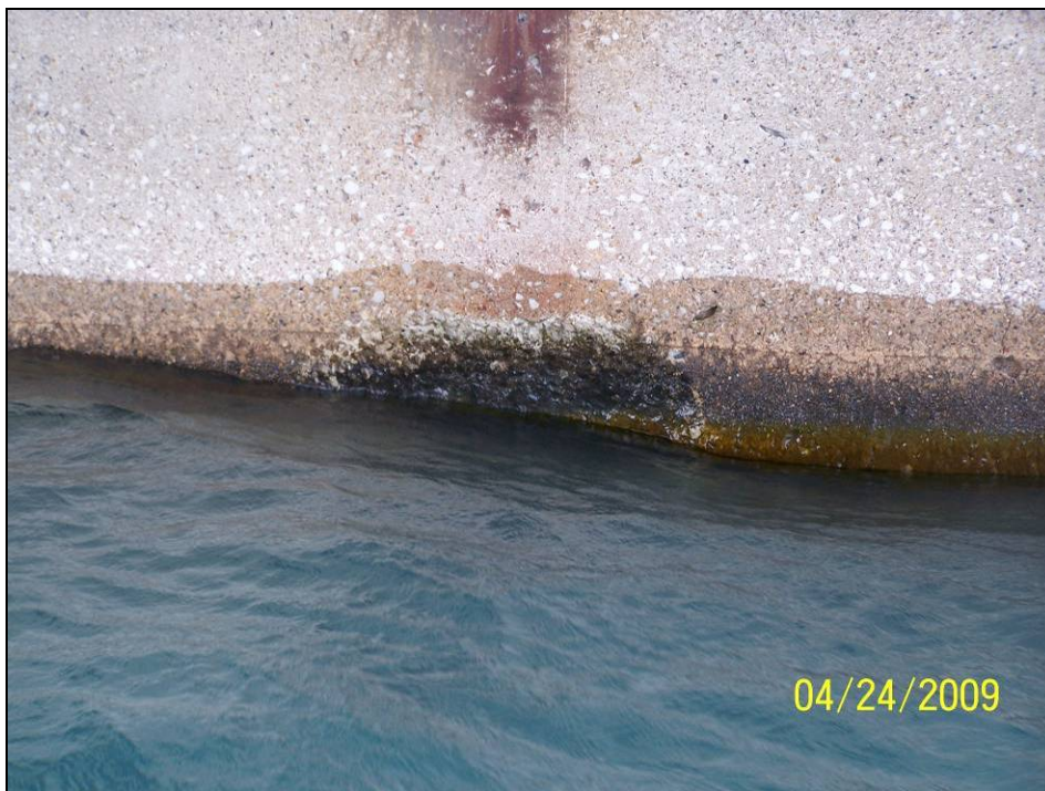
Photograph 98: View of Pier 11 Section Loss 15 Downstream of Northeast Corner.
