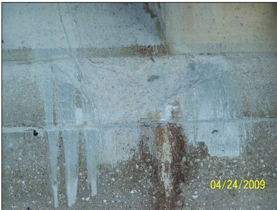
Photograph 92: View of Pier 3 Section Loss on South Face.
