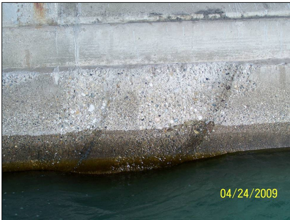
Photograph 104: View of Pier 16 Abrasion Damage on South Face.
