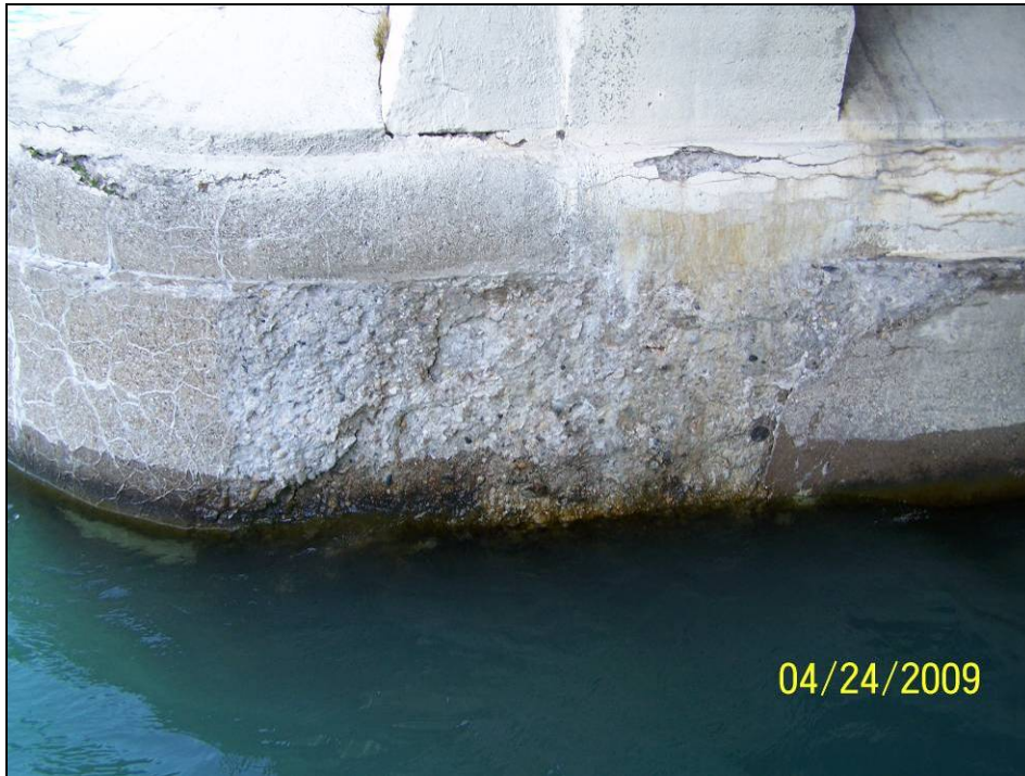
Photograph 105: View of Pier 17 Section Loss on South Face.
