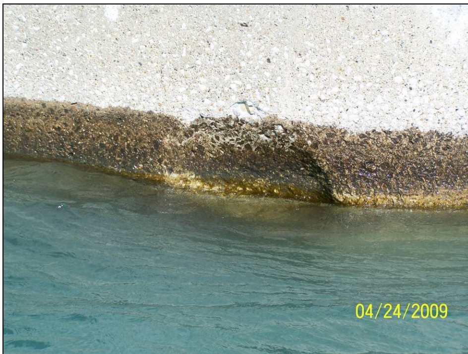
Photograph 100: View of Pier 12 Section Loss on North Face.
