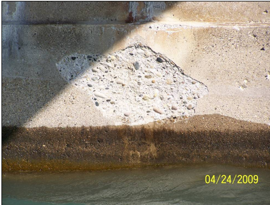
Photograph 91: View of Pier 2 Section Loss on South Face.
