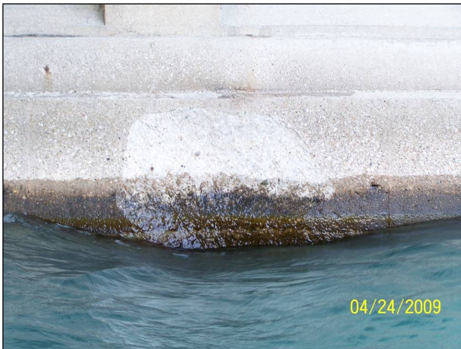
Photograph 102: View of Pier 13 Section Loss on North Face.
