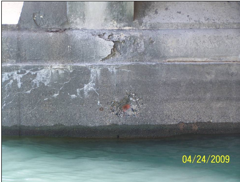
Photograph 89: View of Pier 1 Section Loss Near Northeast Corner.
