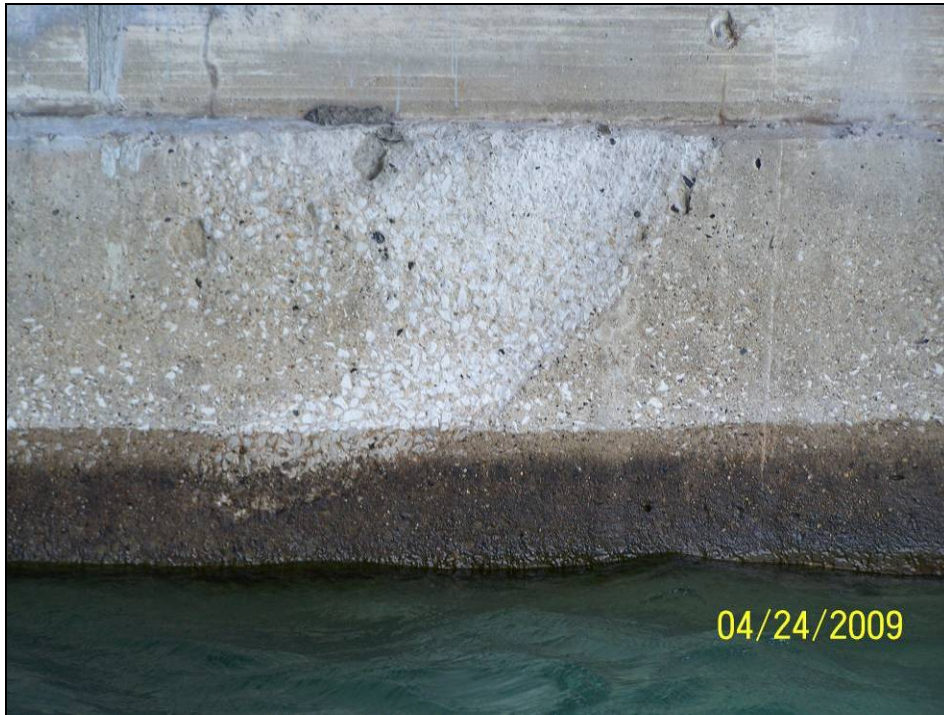
Photograph 101: View of Pier 12 Abrasion Damage on South Face.
