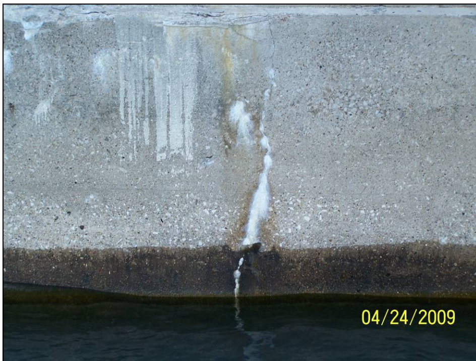
Photograph 94: View of Pier 7 Vertical Crack Near Northwest Corner.
