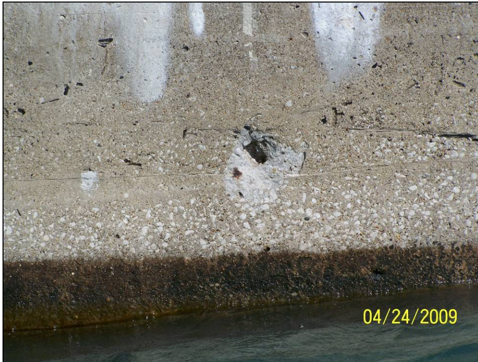
Photograph 95: View of Pier 7 Section Loss on South Face.
