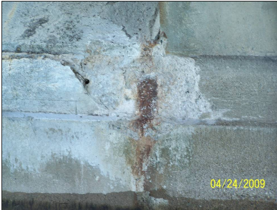
Photograph 103: View of Pier 15 Section Loss on North Face.
