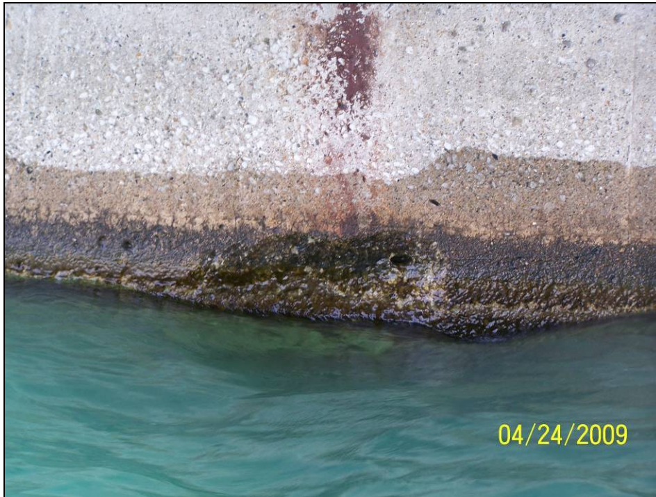
Photograph 99: View of Pier 11 Section Loss 15 Feet Upstream of Northwest Corner.
