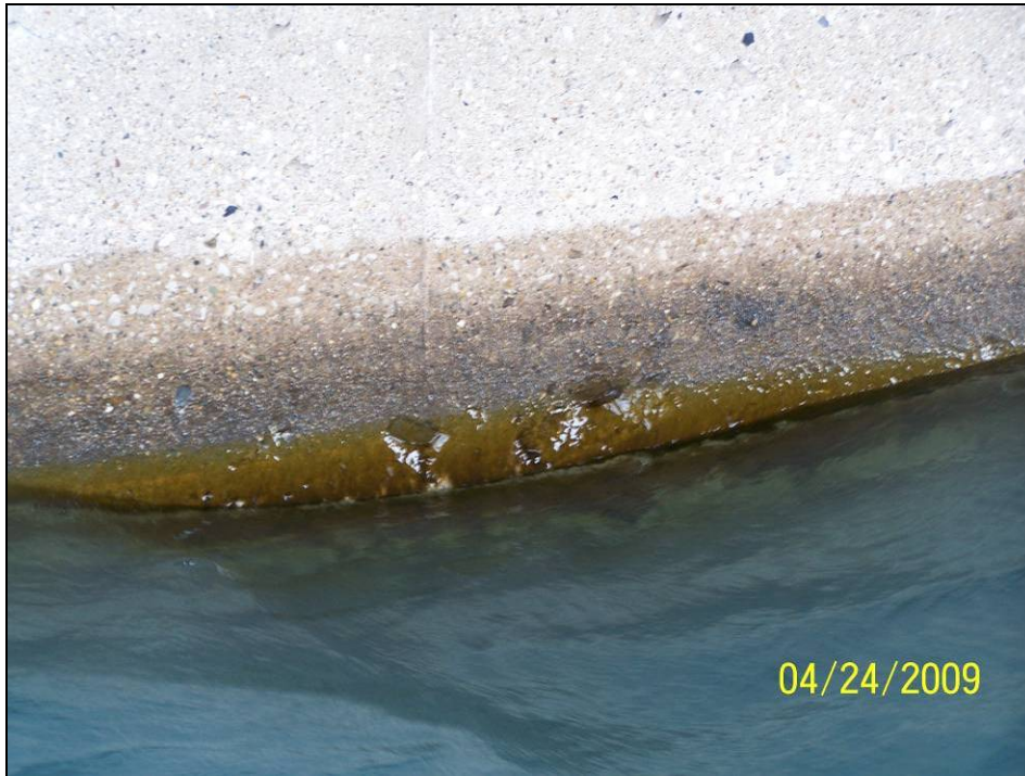
Photograph 87: View of Small Areas of Section Loss Near the Waterline.
