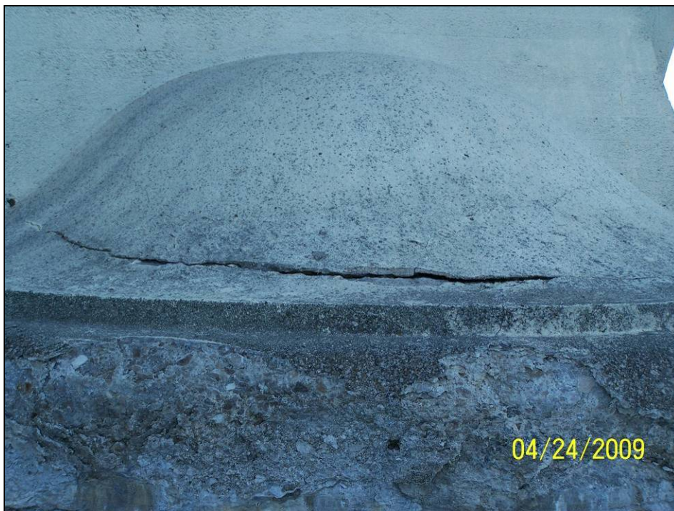
Photograph 96: View of Pier 8 Horizontal Crack on Downstream Decorative Cap.
